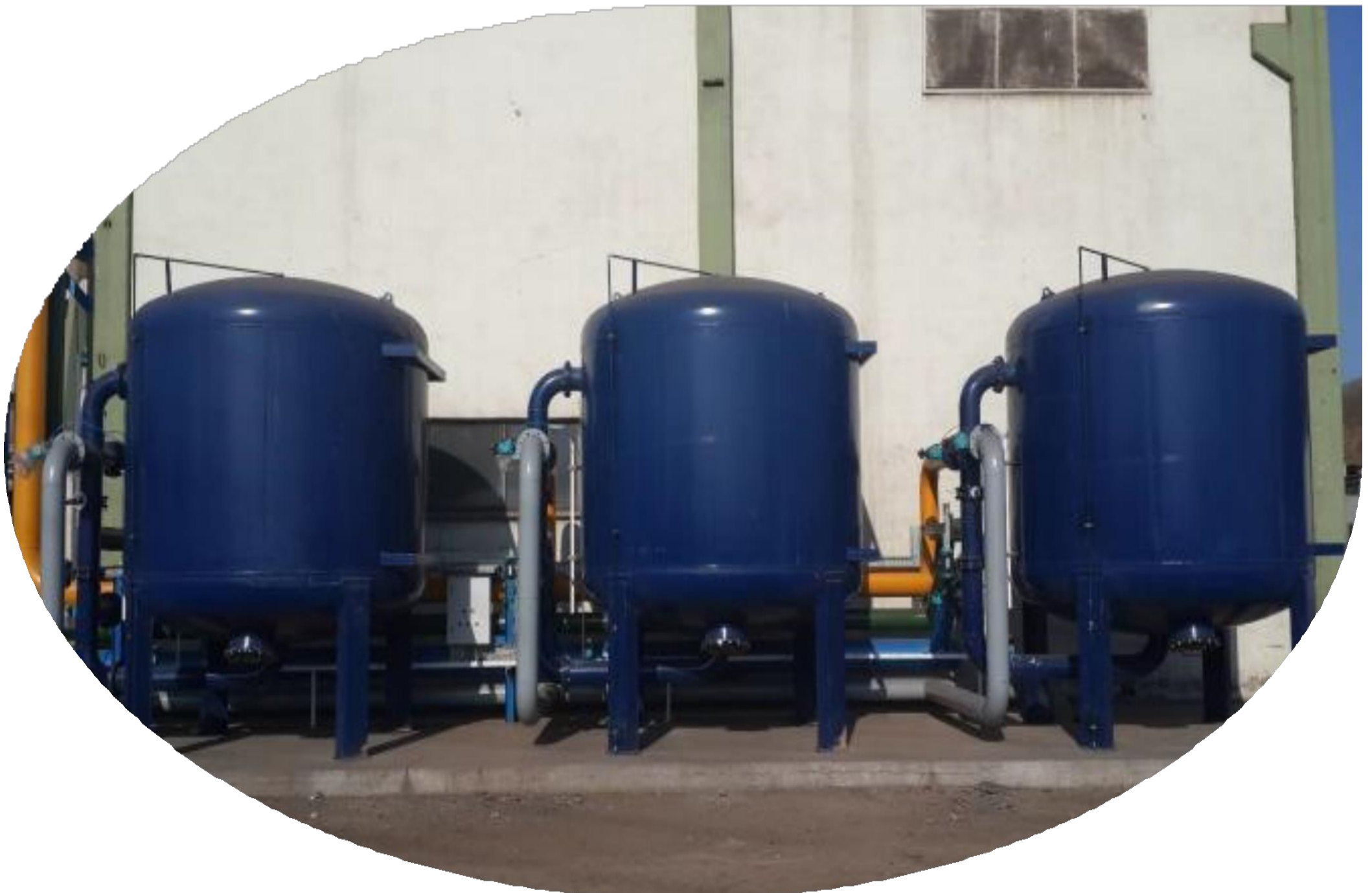
SIDESTREAM FILTRATION SYSTEM 500 m 3 / h
