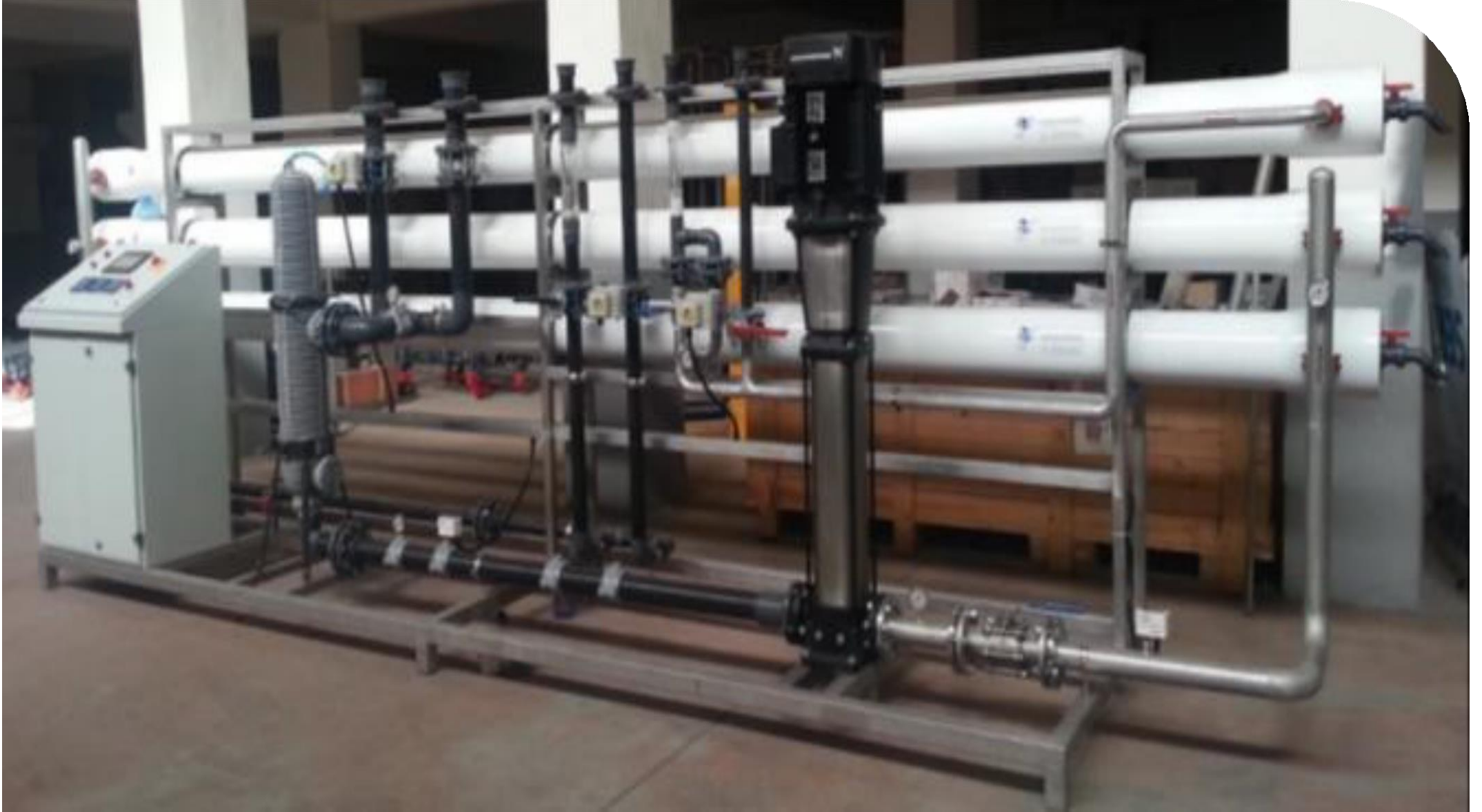
Capacity : 480 m 3 /day REUSE OF WASTE WATER
